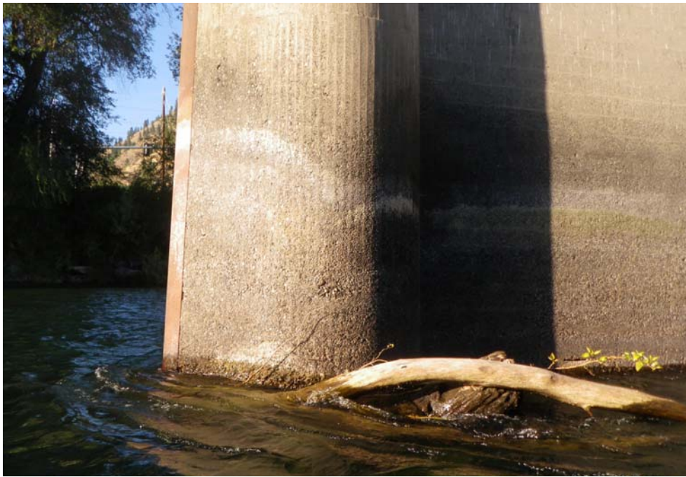
PHOTO No. 3: Pier 5, Looking North - Inspection of the leading edge of the pier found the steel plate to be well secured and evidence of minor abrasive scale on all concrete surfaces exposed to flow.
