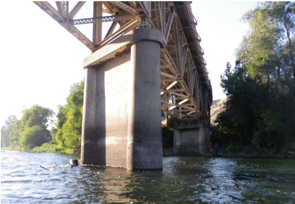
PHOTO No. 1: West Cashmere Bridge, Looking Northwest - Note the build-up of timber debris on the upstream nose of Pier 5 and the minor abrasive scale evident from the high water mark down.
