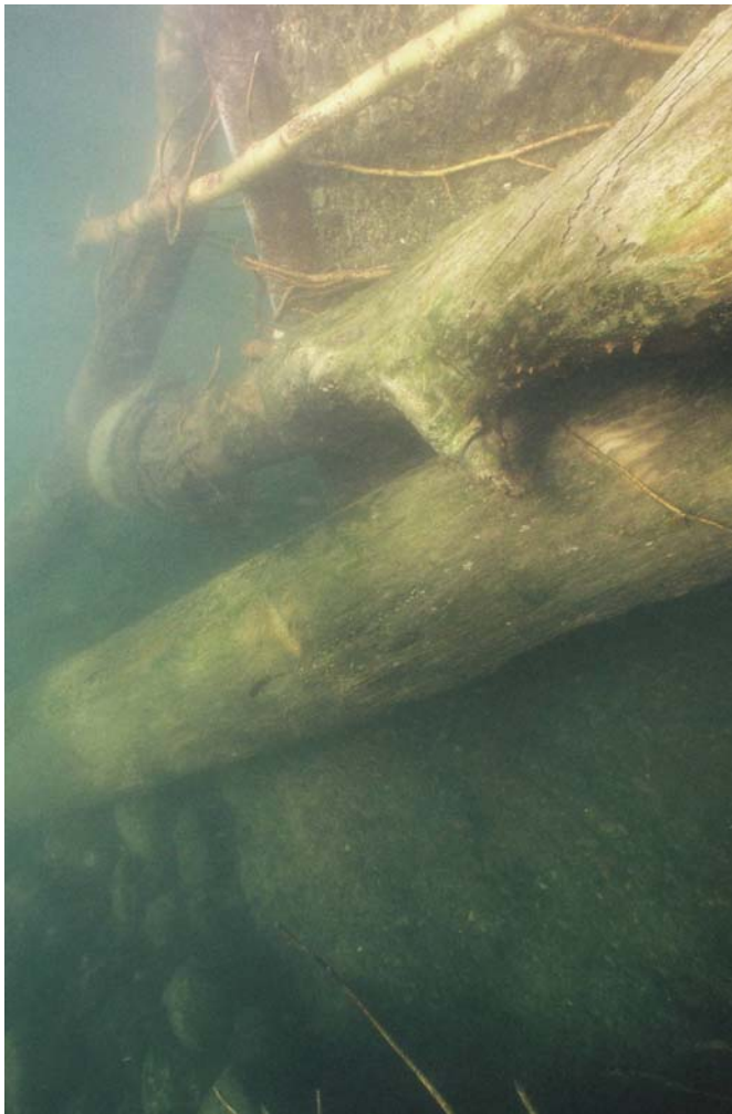
PHOTO No. 7: Pier 5, Upstream End - Note the embedded steel nose plate behind the build-up of timber debris at the upstream end of the pier. Also note the good condition of the submerged concrete and the rock and gravel bottom evident beneath the debris.
