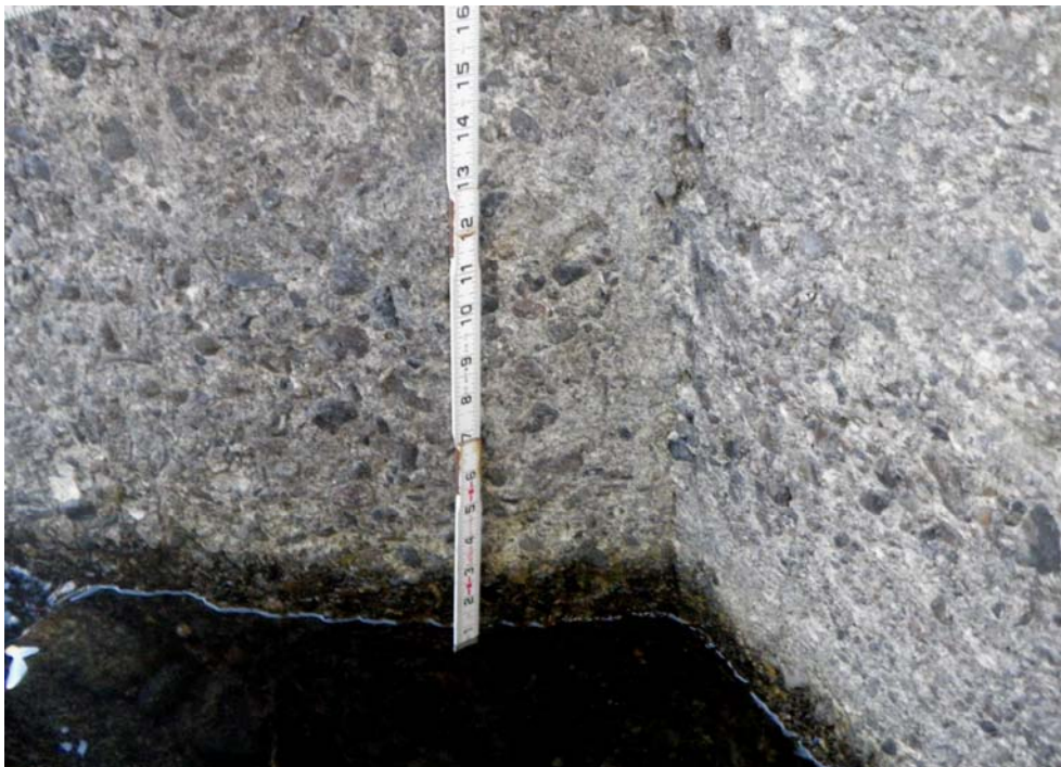
PHOTO No. 6: Pier 5, North Side - Note the good condition of the concrete in this area where the upstream column meets the web wall.
