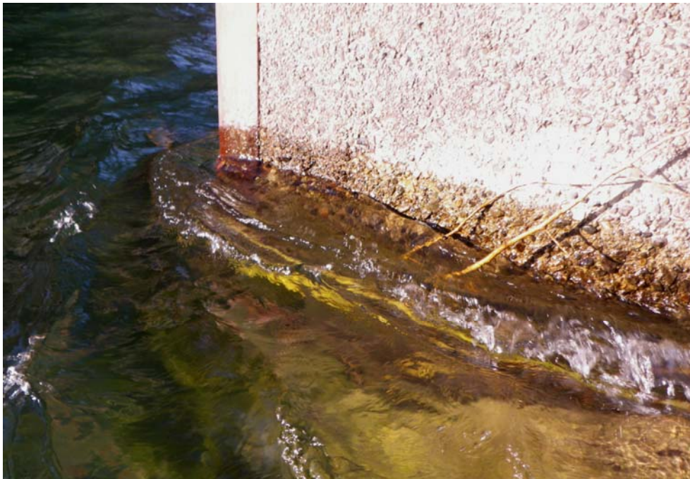
PHOTO No. 5: Pier 5, Upstream End, Close-up - Note the minor abrasive scale at the waterline. This area was noted to have sustained the most significant abrasive scale.
