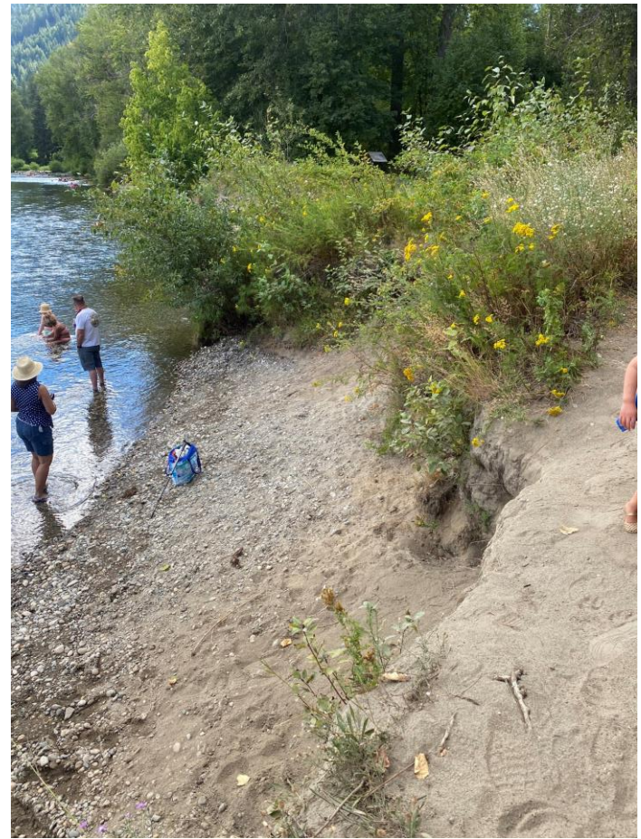
Photo 5 (above): This eroding bank at Enchantment park used to be used for commercial river access.
